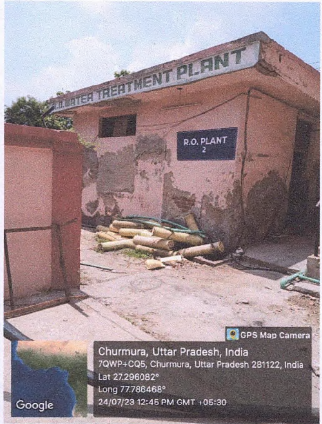
RO Plant-2, HCST
